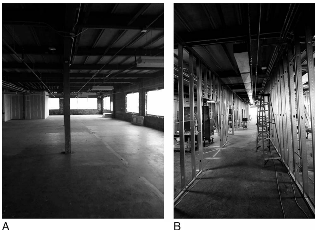
Figure 1. Developed in a former warehouse space, the simulation center began as just an empty shell. The center began to take shape with the installation of wall supports.
